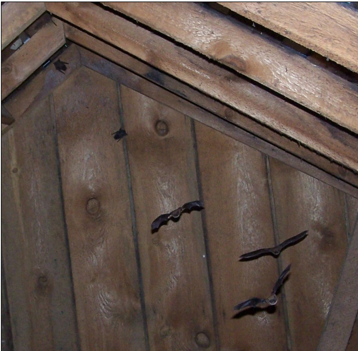
Attic bat roost (Wade Alcock photo)
