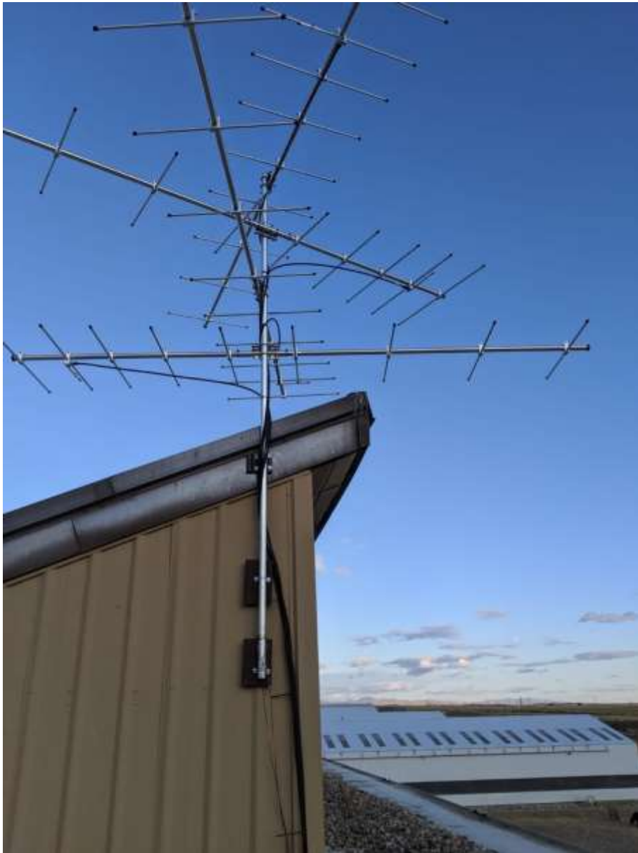
Antennas affixed to metal building. Peregrine Fund Center, Boise, ID.
